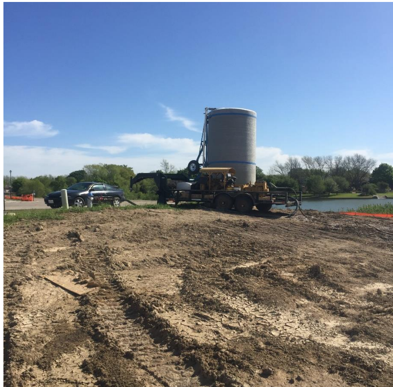
Tank Contains Water and Chemical
